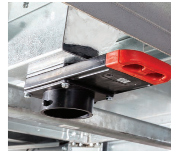
Toilet waste valve.
