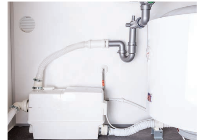
Service room includes a 50L boiler for warm water and a grinder to deal with the waste coming from the sink and toilet. Each bathroom has its own individual boiler and grinder.
