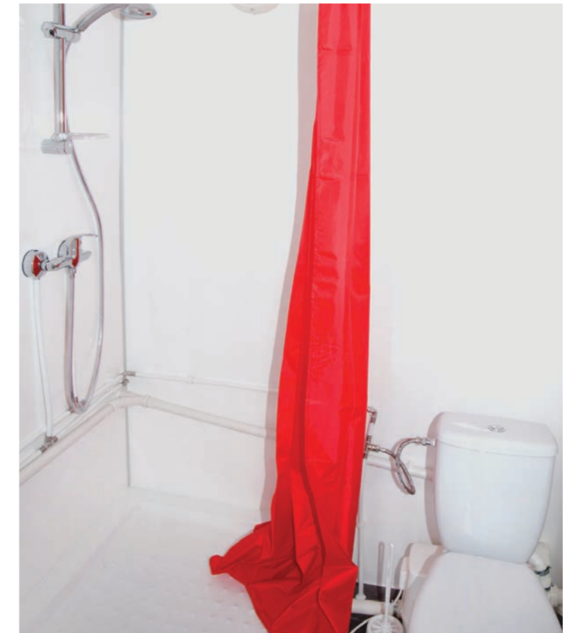
Ceramic toilet bowl, heater, shower, grinder and a boiler in the bathroom. Certified heater to withstand wet conditions.
