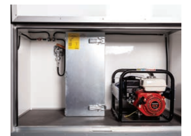
Portable generator and gas tank locker.
